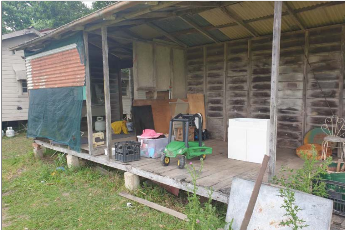
Photograph 5: Dilapidated outhouse/shed with corrugated fibre cement & iron roof and possible internal cement sheeting (potentially containing asbestos) (17 November 2020).
